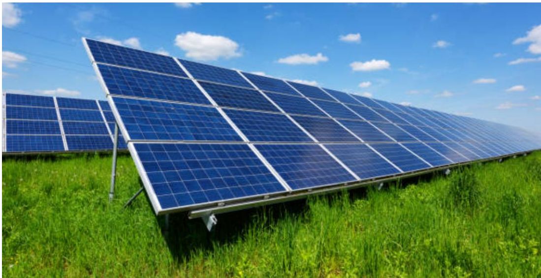
Figure 13: PV farm in India (www.constructionworld.in, 2022).
