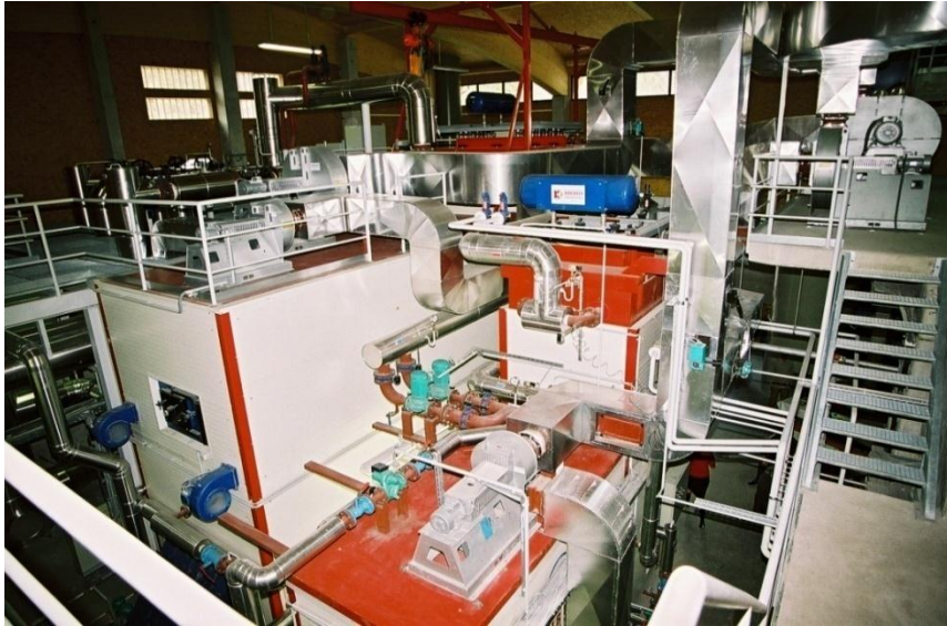
Figure 24: Boiler plant incl. heat exchanger and parts of flue gas cleaning
