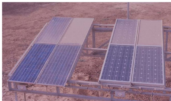
Figure 27: Test arrangement in Dakar
