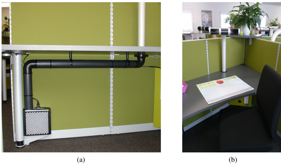
Figure 2.9: (a) Ductless PV air intake and (b) PV supply diffuser
