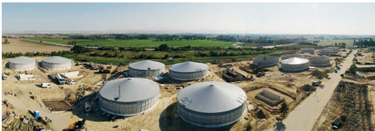
Figure 14: Building site of a biogas digestion plant park based on renewable resources in Güstrow (Germany)
