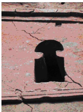
Picture 10, tensile cracks on the Bete Medhane Alem
