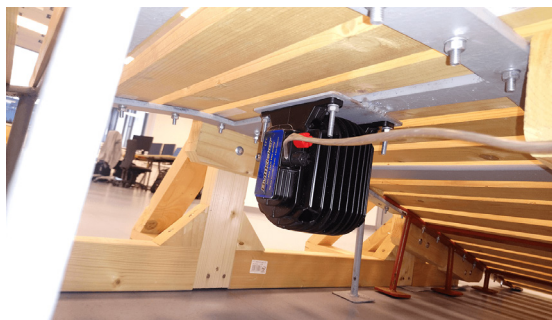
Figure 4.5: Supporting welded steel arch structure and audio transducer mount on the underside of the curved bridge prop.
