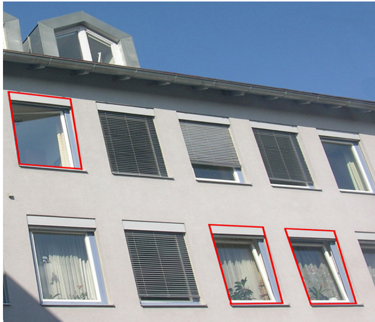
Figure 2.2-10 Opened and tilted windows
