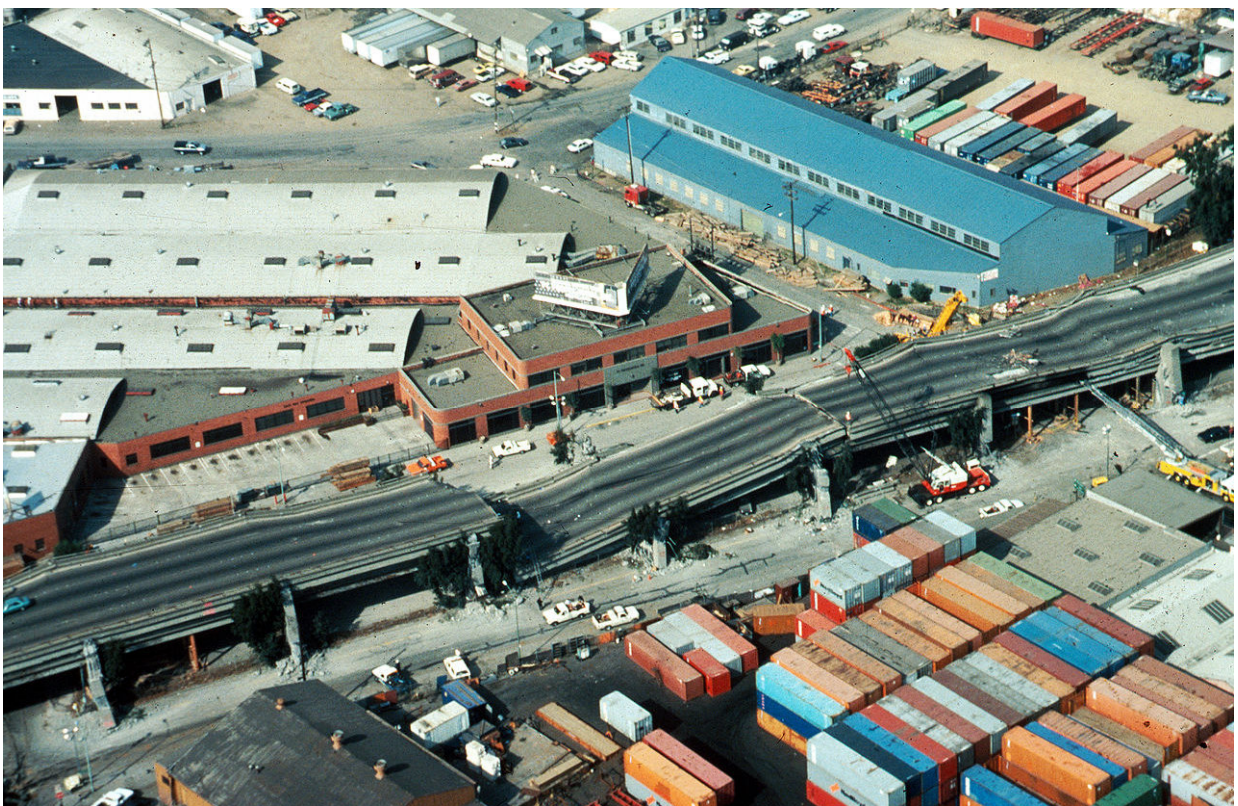
Figure 44: Image of collapsed double-decker freeway structure in Oakland, California [54]
