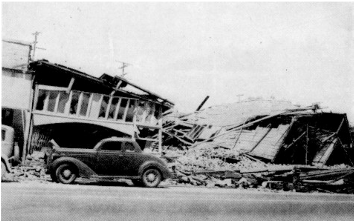
Figure 42: Collapsed buildings in Imperial, California, in which four people died [52]
