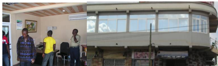
Fig.15: Exposed glassing on the western façade
