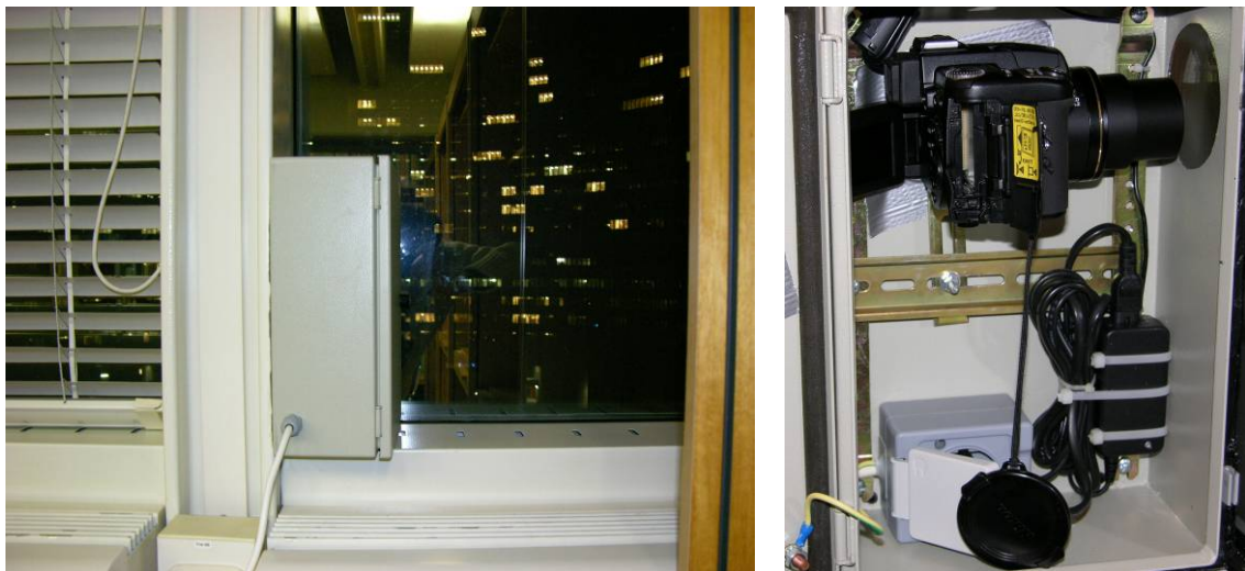
Figure 2-27 Camera case mounted indoors in VC pointing to VC-N façade and close-up of the camera case.
