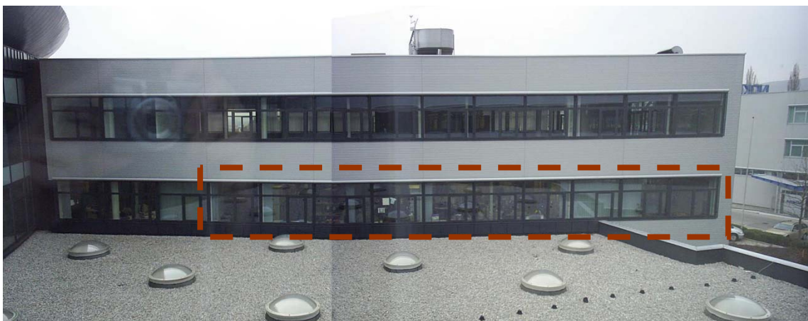
Figure 2-26 Observed area of ET façade, picture stitched out of the two webcam perspectives
