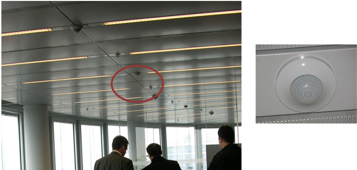
Figure 2-24 Illuminance sensor, mounted on the ceiling in UT and close-up
