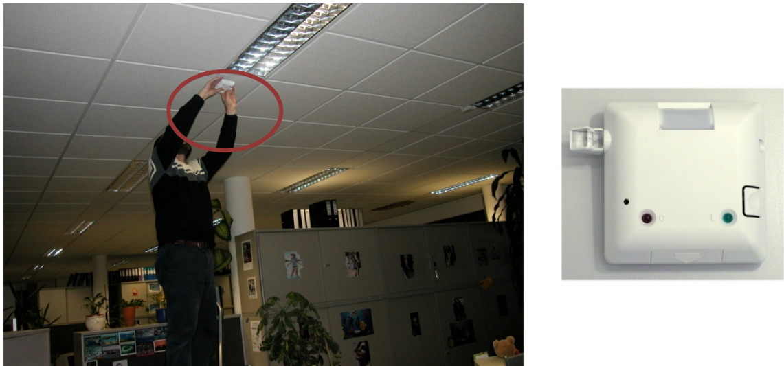
Figure 2-25 IT-200 loggers mounted on the ceiling in ET and close-up
