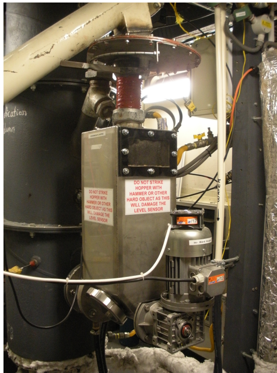
Figure 6.17: Intermediate hopper and in-bed auger in Christchurch/NZ
