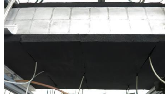
Figure 17: Armaflex (3,2 cm) is used to insulate the whole RPW-HEX.
