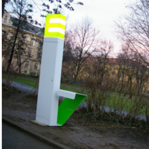
Picture 16: e-power station in Klagenfurt Source: "lebensland Kärnten", 2009 (14. Oct. 2009)
