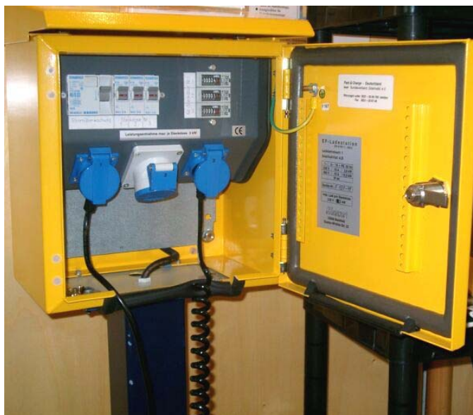
Picture 18: Typical „Park & Charge“ Station (three phase connection, 2 x isolated ground receptacle and 1 x CEE socket with FI-switch, 3x 16A fuse)
