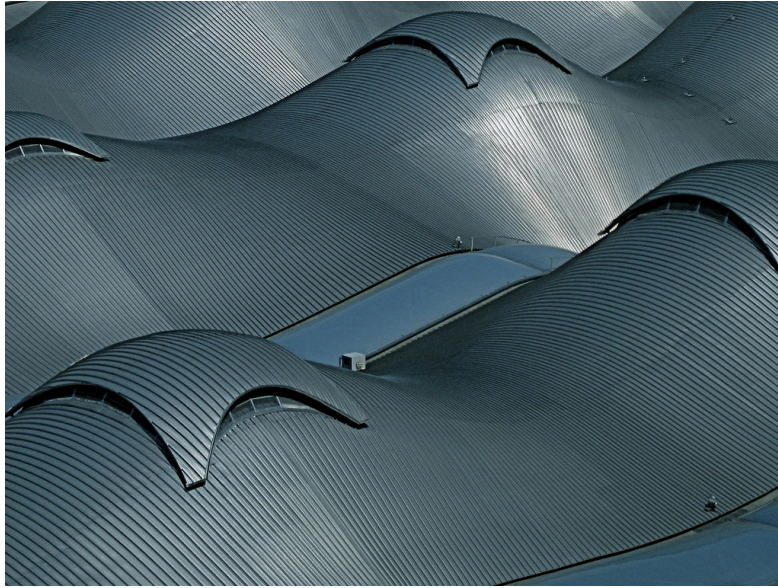
Figure 2.1: The roof of Southern Cross Station at Melbourne, Australia, covered with straight metal panels. Photo by Dale Gillard via Flickr.
