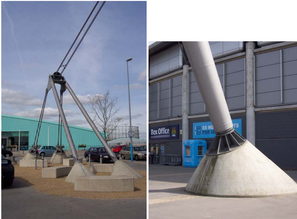
Fig. A-6: left: foundation of the corner ties that form the grounded tension ring; right: foundation of the cigar-shaped mast
