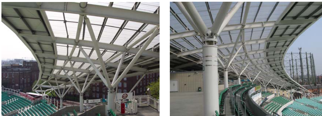
Fig. A-3: Roof structure of the OCS Stand with supporting trees and cantilever beams
