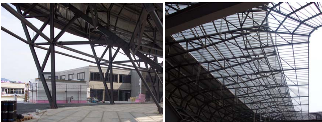
Fig. 3.5: left: Concourse level with temporary steel element at the back; right: Roof trusses above the temporary second tier with a temporary roof extension at the front
