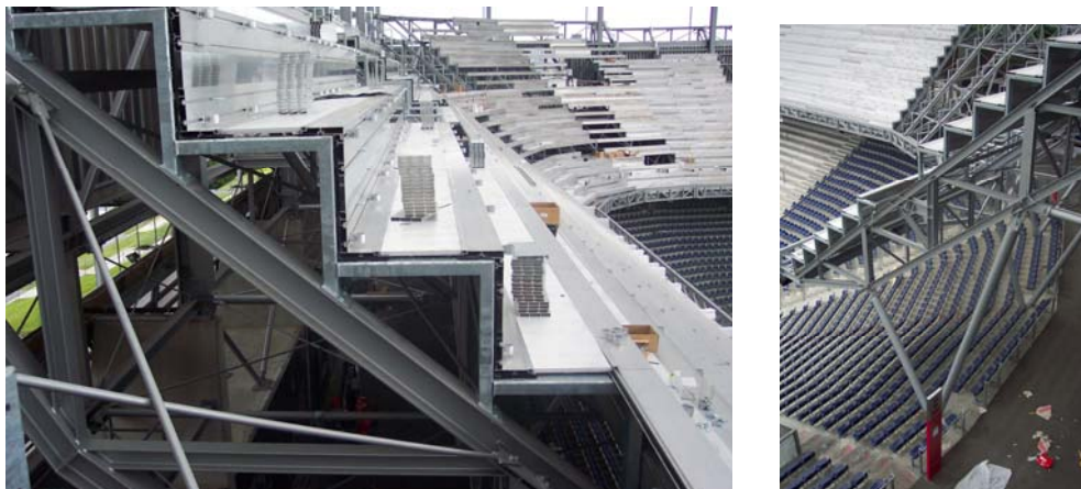
Fig. 3.7: left: Detail of rakers and seating elements of the temporary upper tier; right: Rafter and V-column of the temporary upper tier
