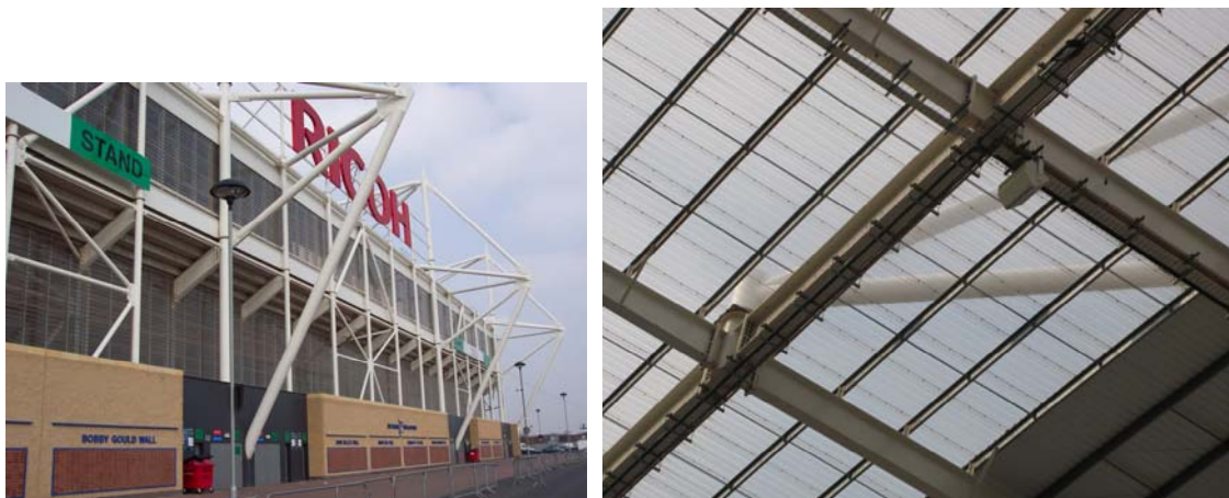
Fig. A-44: left: Stadium façade; right: Detail of the connection between stays and roof frame
