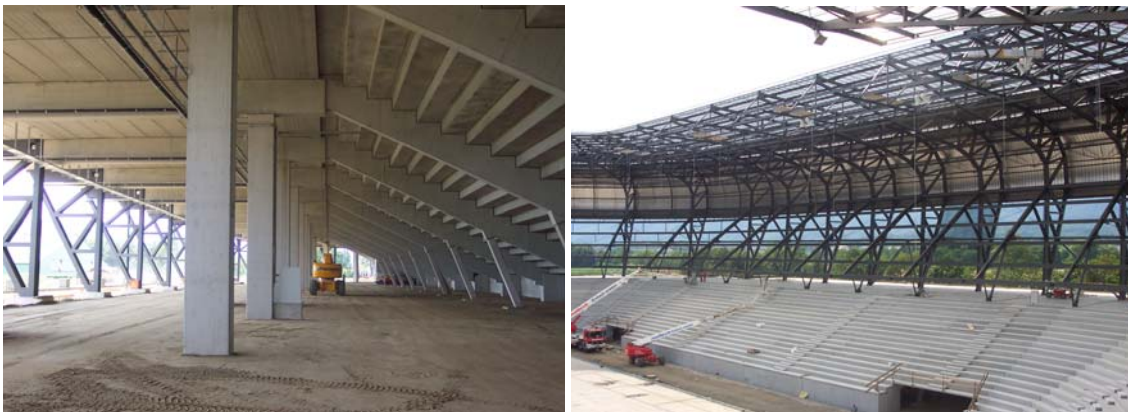
Fig. 3.4: left: Permanent concrete structure of lower tier; right: Temporary upper tier and roof
