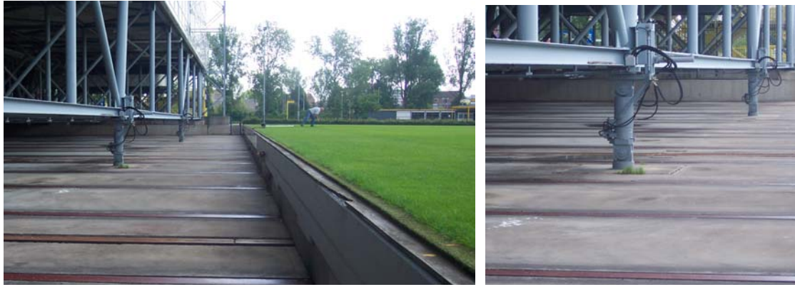
Fig. 3.23: Gelredome : temporary props for the stand structure and the pitch outside the stadium
