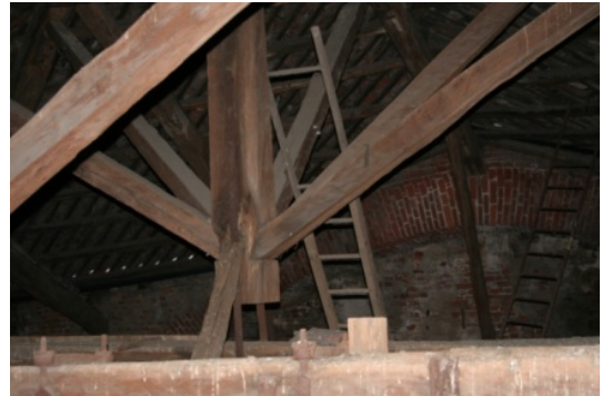
strut to overtake the forces coming from the umbrella structure (bearing on the vault)
