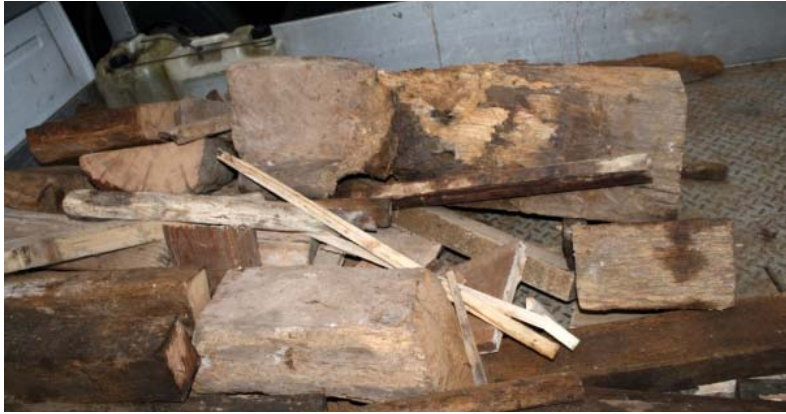
Illustration 56 Element, which had been substituted
