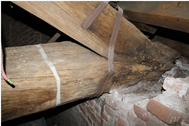
Illustration 41 Damaged tie beam
