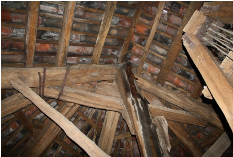
Illustration 40 Water infiltrations on the peak
