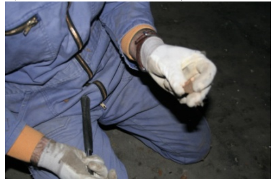
sample of weakened timber (hammer)
