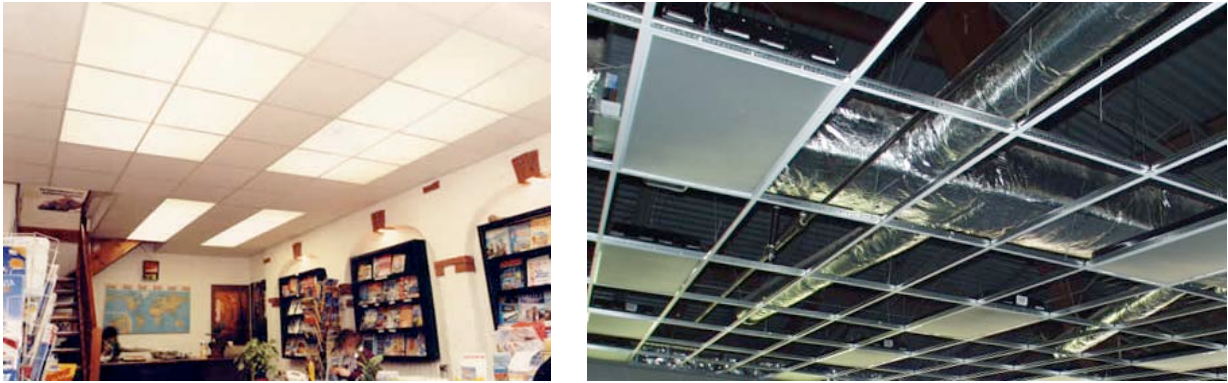
Figure 2.14: Dropped ceilings made of metal grids clad with lightweight tiles – containing light fixture elements (left) and used to conceal piping, wiring, and ductwork (right).
