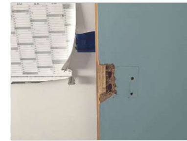
42. Damaged door after removal of metal hardware (2022)
