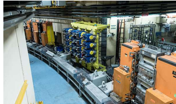
(b) The new PSB injection system during the installation phase in 2019, displaying the 16 BSW magnets (4 per ring) in blue [93].
