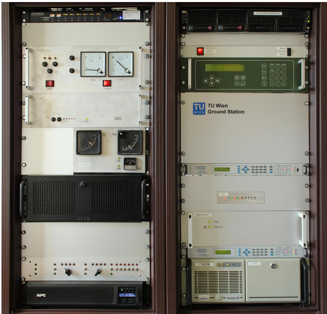
Figure 7.1: Photo of the TU Wien Ground Station's indoor components.
