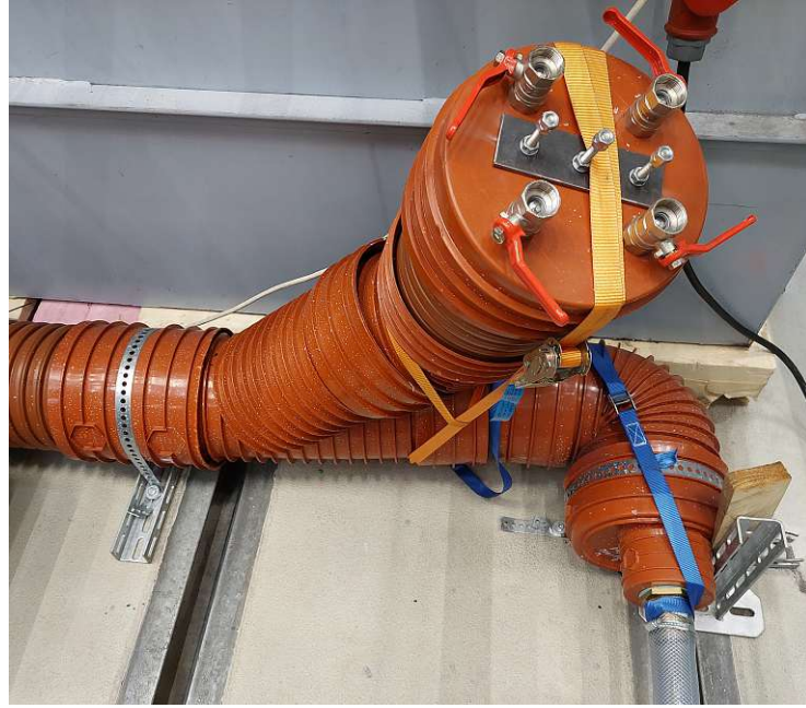
Figure 29.: Bypass valve in air supply line.
