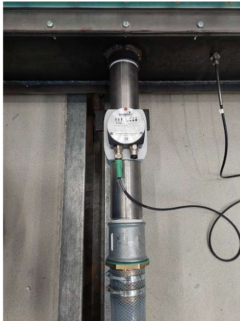
Figure 32.: Built-in volume flow sensor IL30.020.
