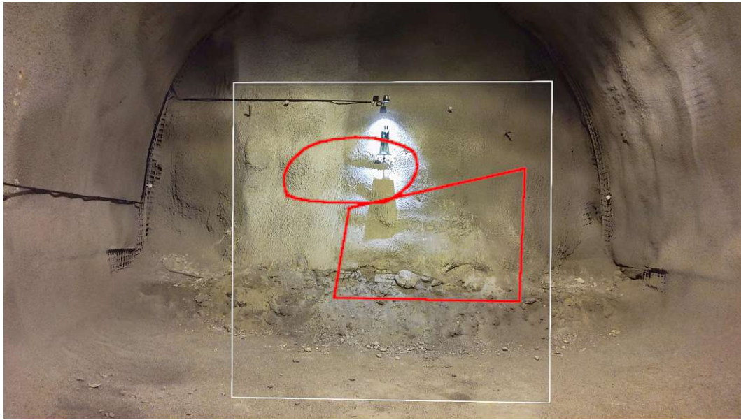
Figure 2.3: An example of a tunnel face mapping captured during the usability test.
