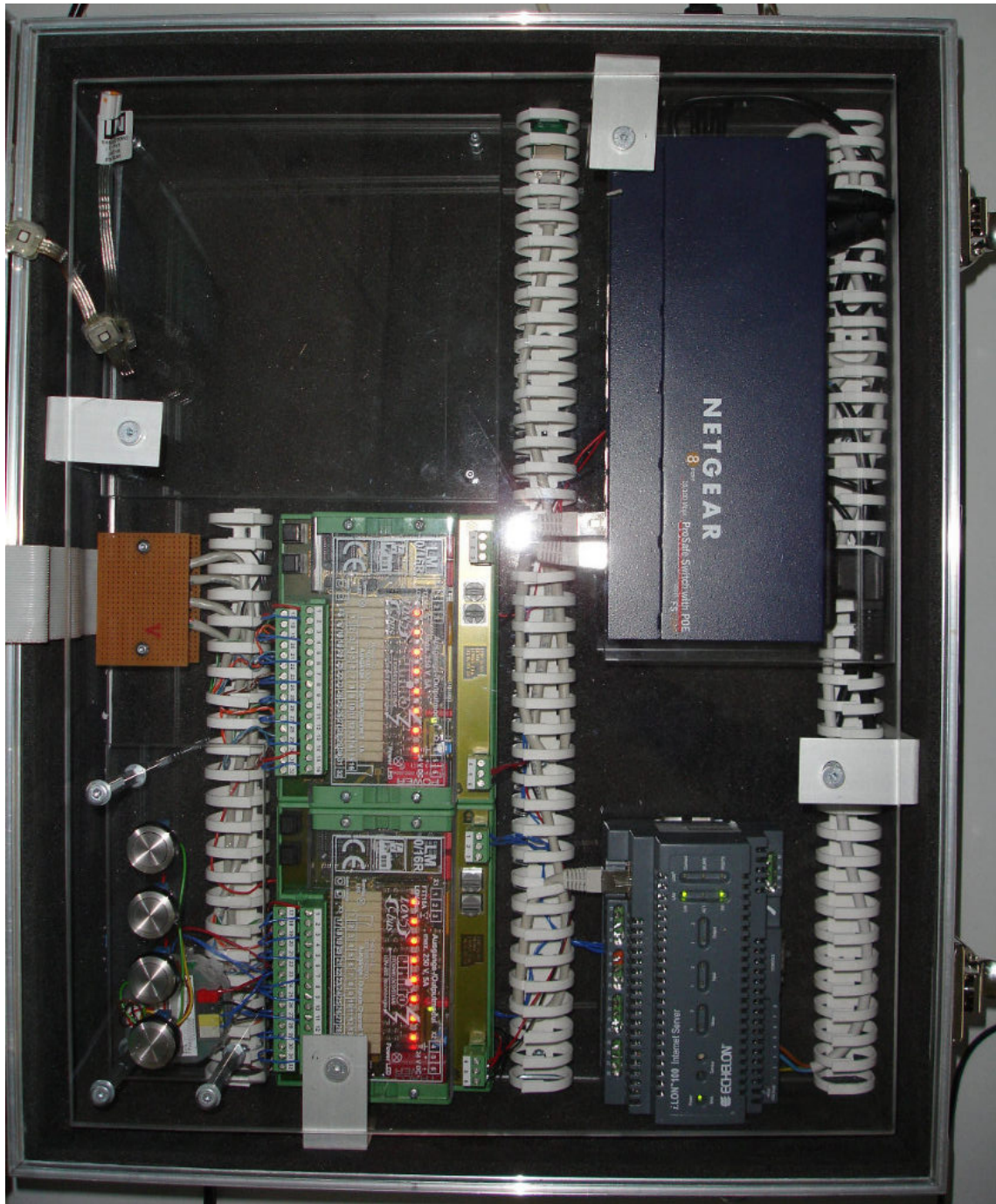
Figure 6.6: Picture of the components of the demonstration suitcase. At the bottom of the picture the i.LON 100 resides on the left the Ethernet switch on the right side. At the top on the left the LonWorks input and output modules and the push-buttons are visible. The Image Generator would be located at the free space in the upper right corner, but is missing in the picture.
