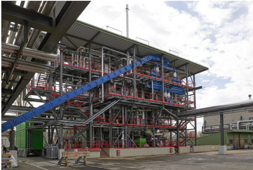
Figure 2.2: 1 MW DFB steam gasification plant in Simmering with project name Waste2Value by BEST-research[21]
