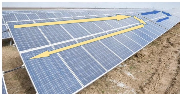
Figure 6: String cabling for OWL, C - Style (own design, picture Active Solar)
