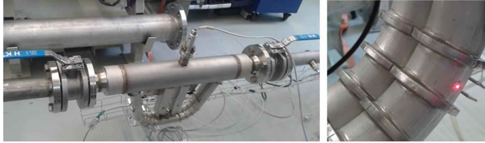
Figure 5.6: A dual-channel mass flow meter installed in the calibration rig and the laser vibrometer measurement points at the sensor positions for the displacement measurement.
