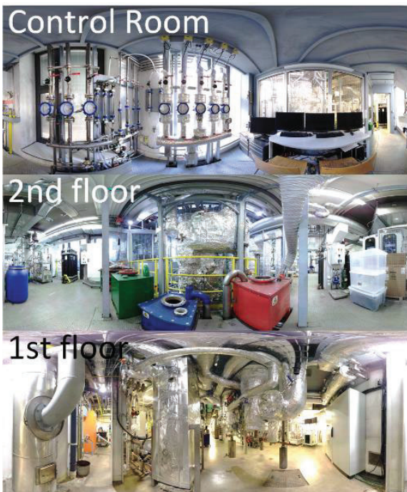
Fig. 4: Picture of the control room, 2 nd floor and 1 st floor of the advanced 100\text{ kW}_{th} pilot plant
