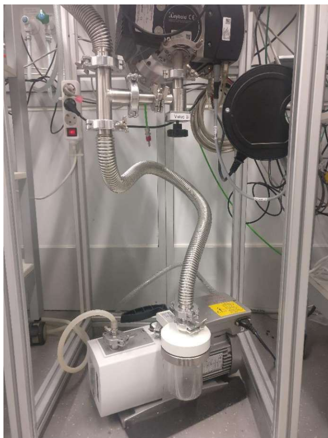
Figure 38: Vacuum backline, showing the TMP and the rotary vane pump, connected by a T-piece. By opening of a bypass valve (outside of picture) the chamber can be evacuated by the backing pump directly, without passing the TMP. This minimizes the risk of particles falling into the TMP when evacuating at atmospheric pressure.
