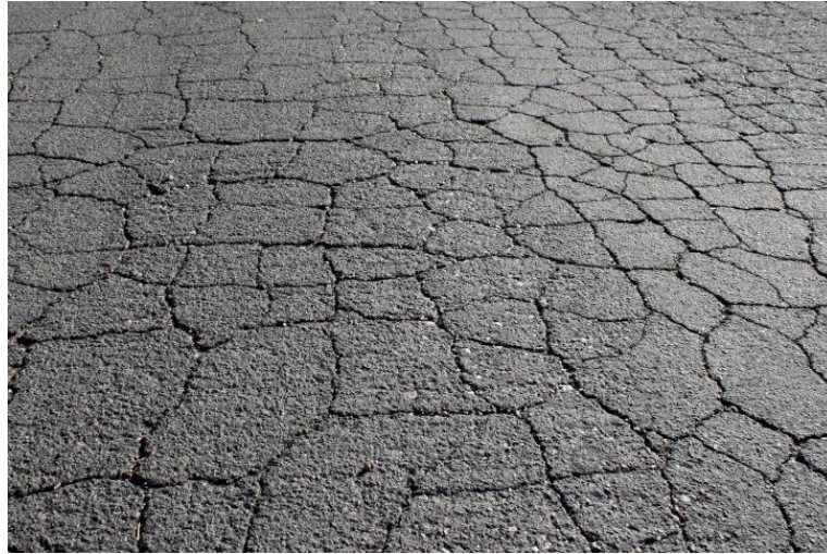
Figure 2: Possible cracks in asphalt during its service life on the roads [9]
