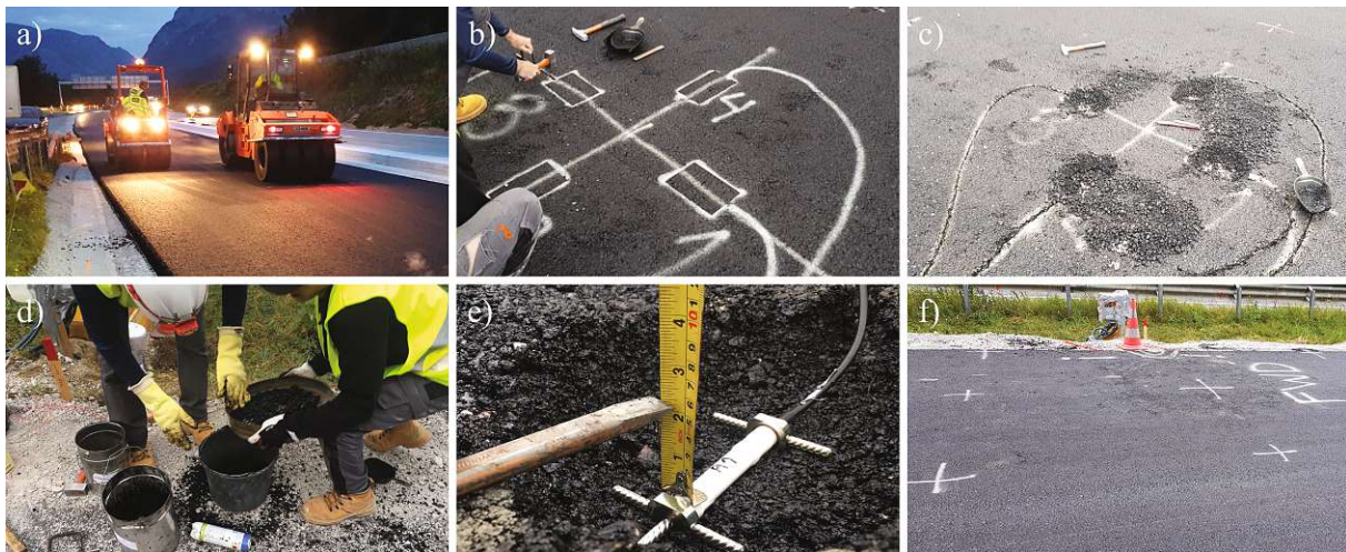
Fig. 4.9. Installation of asphalt strain gauges at field-testing site #1 on the A10 using method A: Cut, install, and cover after asphalt placement.
