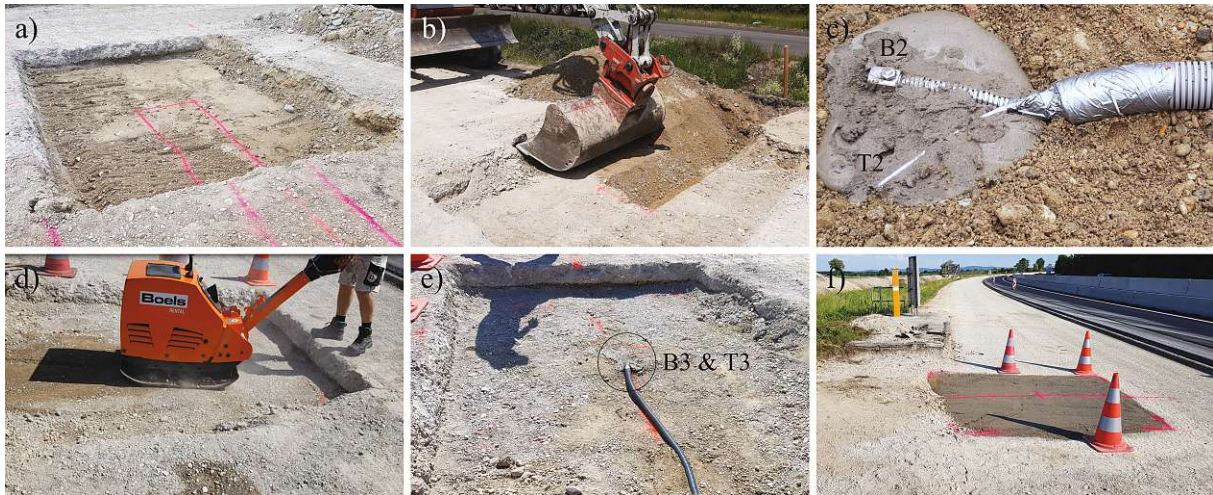
Fig. 4.4. Installation of accelerometers in unbound granular layers on the motorway A3: (a) excavation of the cement-stabilized layer, (b) smaller excavation of the unbound layer down to its boundary with the subgrade, (c) installation of sensors at the surface of the subgrade, (d) refilling and compaction of granular material, (e) installation of sensors at the surface of the unbound layer, and (f) placement of lean concrete.
