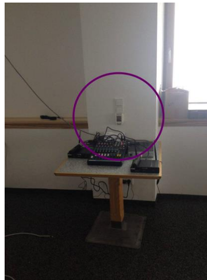
Figure 37. Seminar Room Measuring Location 1. Multi Sensor (Temp, RH and CO 2 ) Device 1
