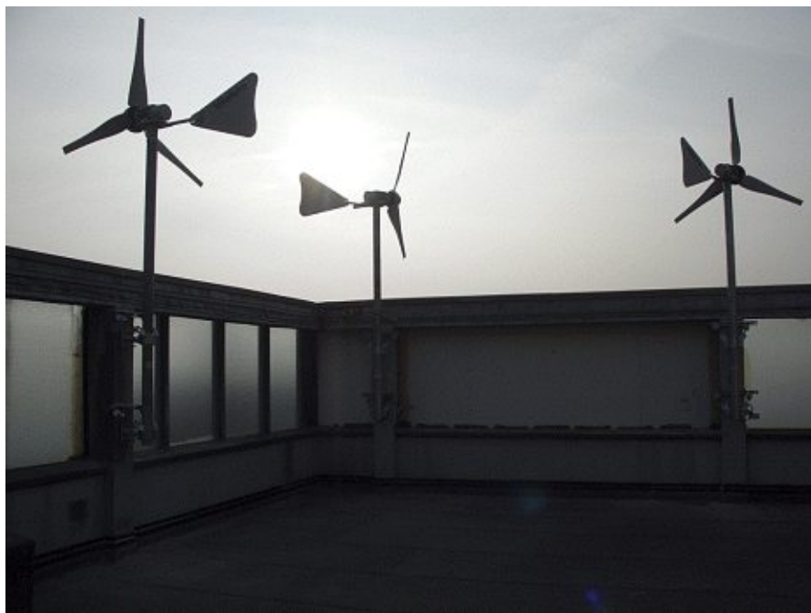
Figure 16 Small wind turbines installed on CIS tower in Manchester, UK (Source: BBC 2005)
