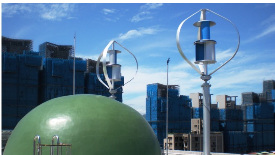
Figure 17 Small wind turbines installed on the rooftop of ROC (Source: Ministry of foreign affairs, Republic of China (Taiwan) 2013)
