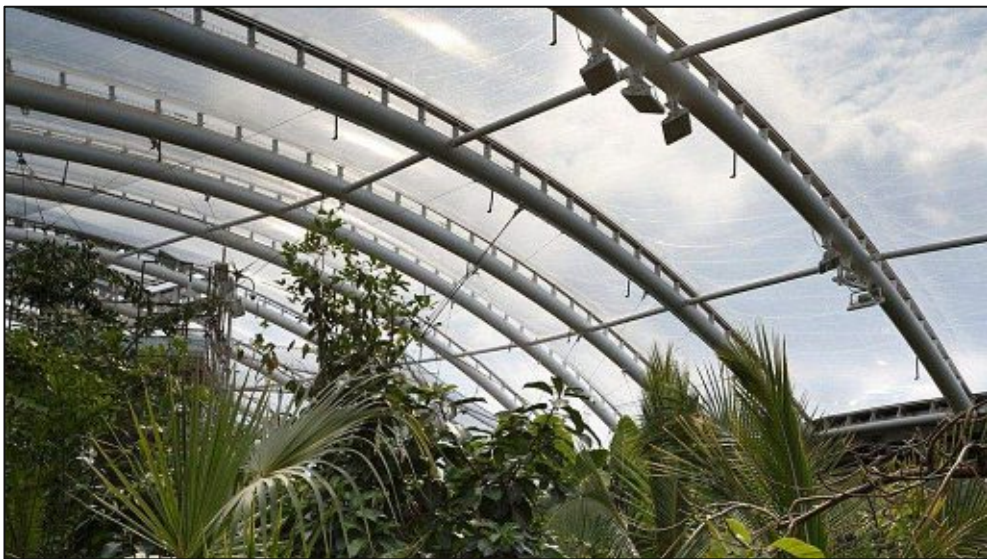
Figure 18: Long arched ETFE cushion roof with interconnecting members and high upstands – Islands at Chester Zoo Building, Chester, England (website: e-architect.co.uk ) 10
