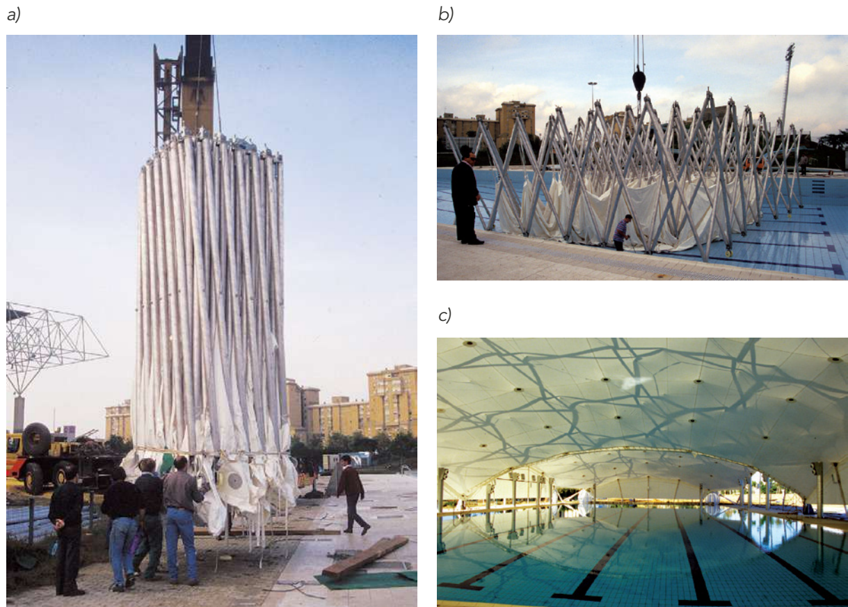
Figure 15: a) Fully contracted structure. b) Deployment process. c) Interior view when fully installed.
