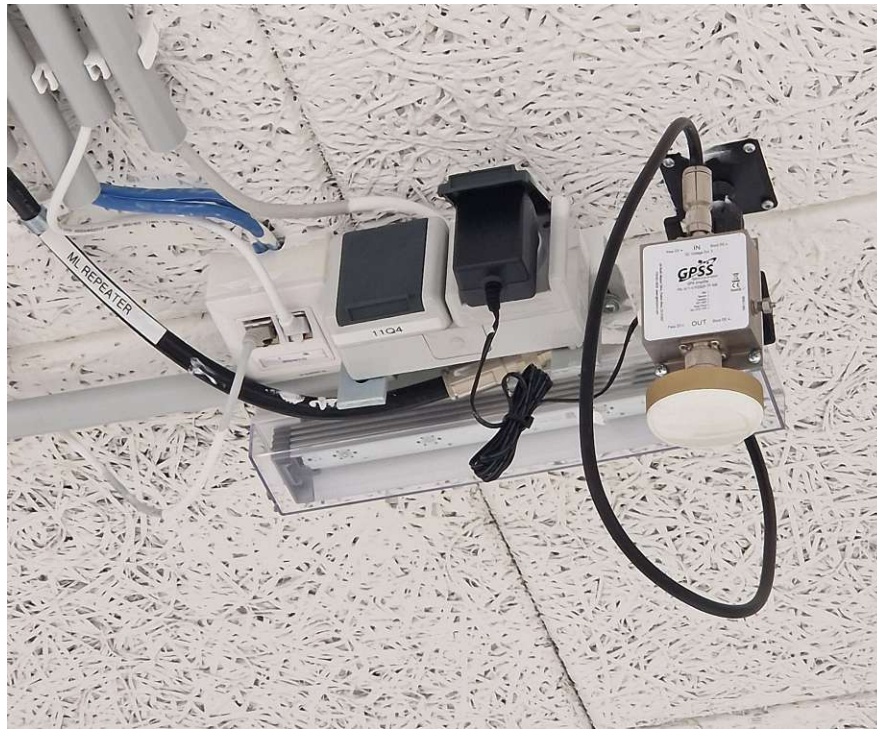
Figure 3.6: GNSS signal repeater on the ceiling of the measurement laboratory
