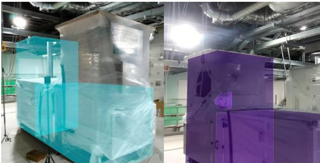
Fig. 29: Identifying mechanical equipment installation errors using Augmented Reality technology.
