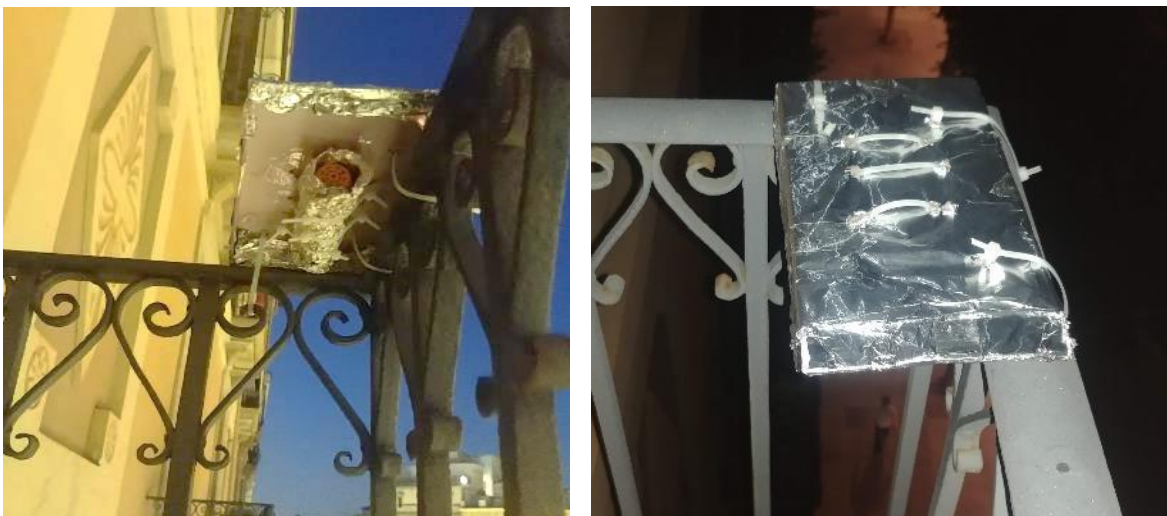
Figure 35. Installation of the sensor-logger
