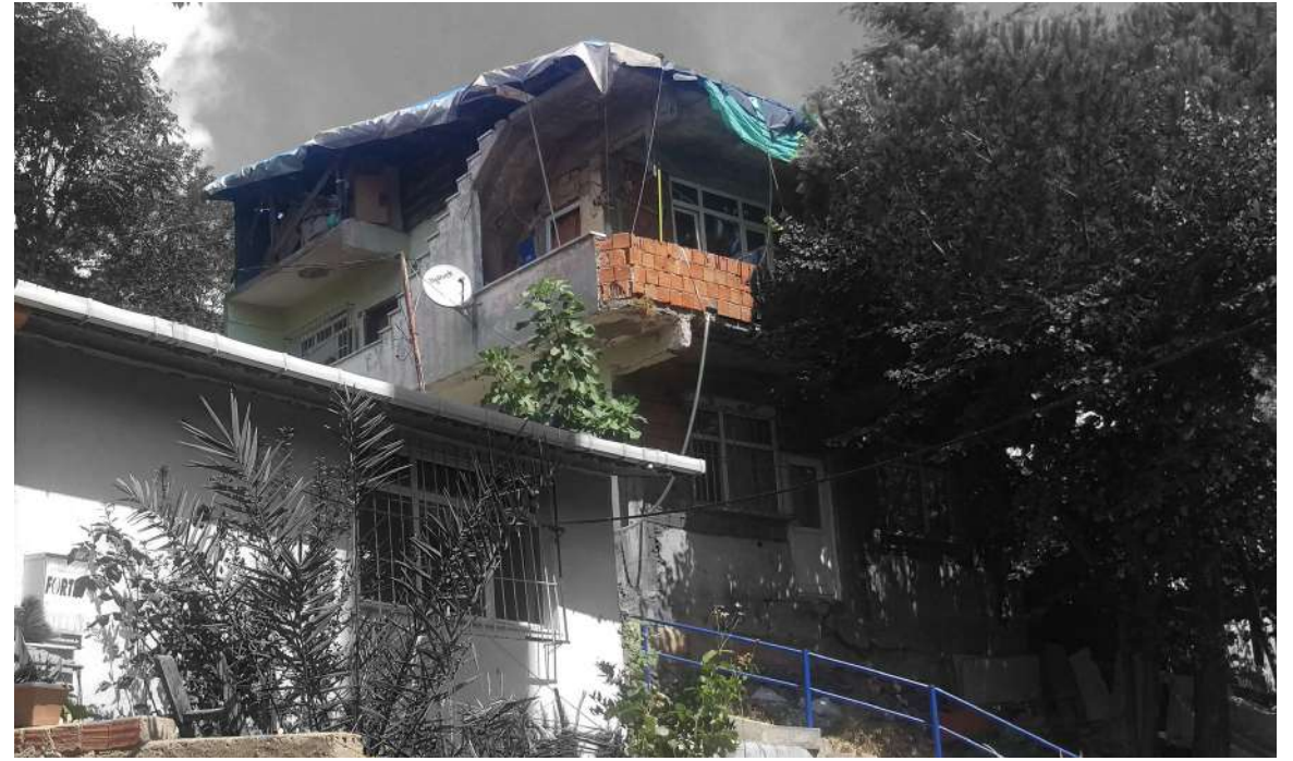
Fig 131 Accessibility problems due to later built vertical expansions and later added stairs for vertical circulation
