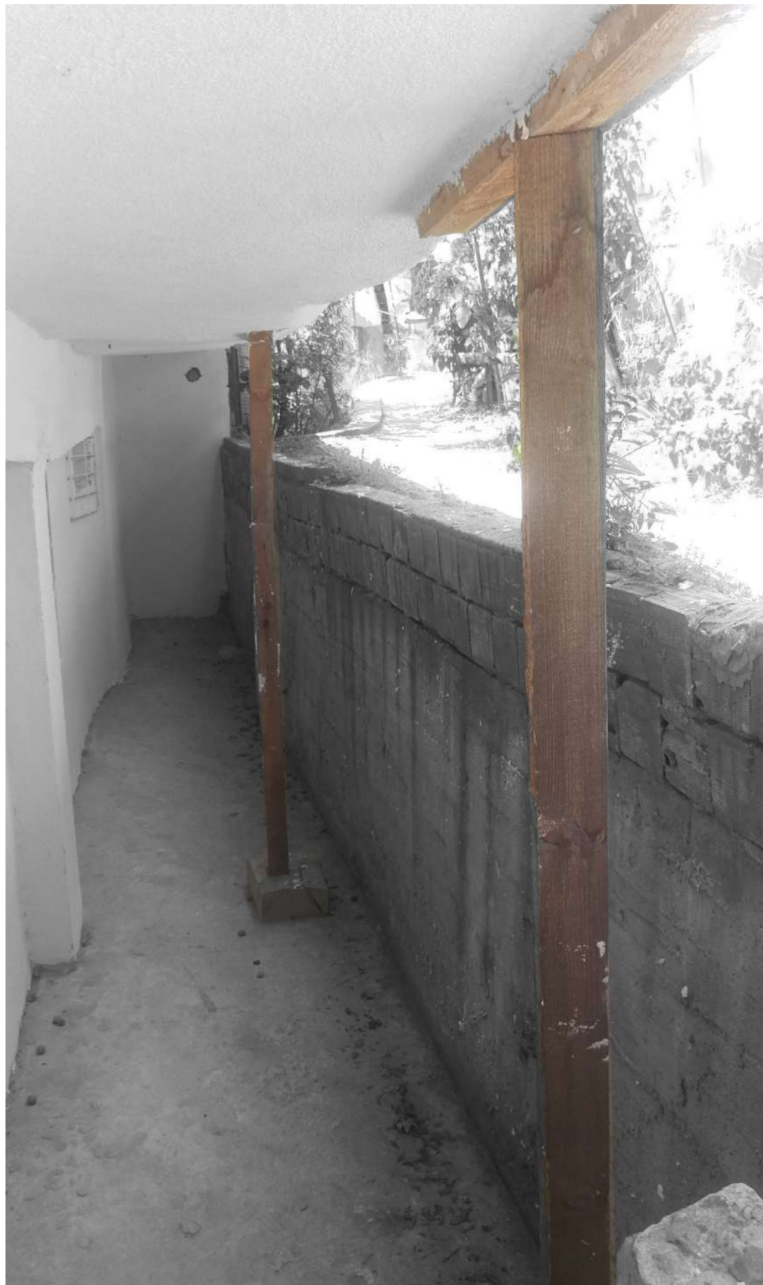
Fig 134 Structural problems due to self-help nature of gecekondus and future expansions
