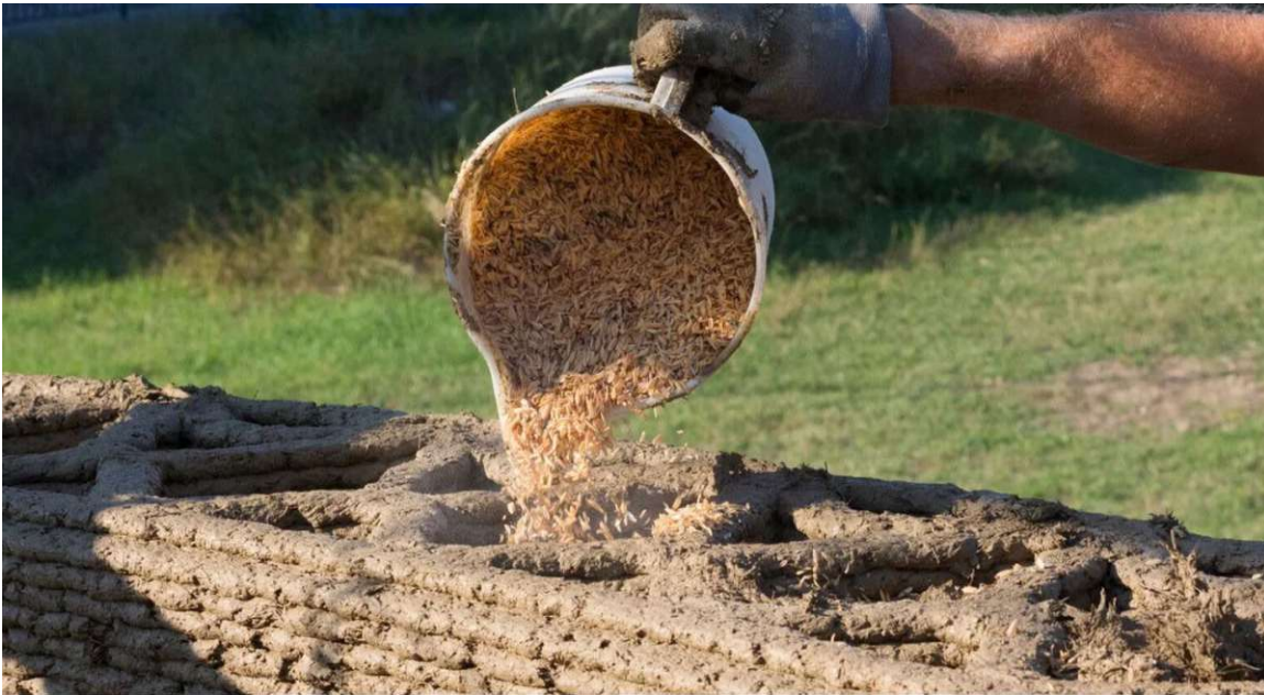
GAIA, Rice House in collaboration with WASP 3D; 3D printed house out of Rice by-products materials
