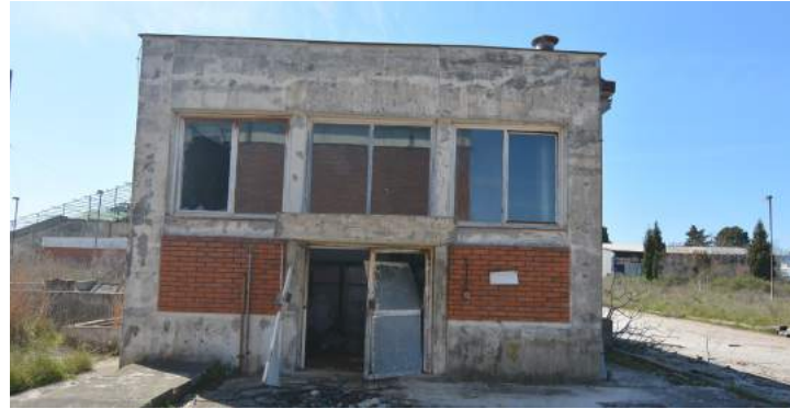
Fig.69 Unit for unloading, storage & transport of heating oil
