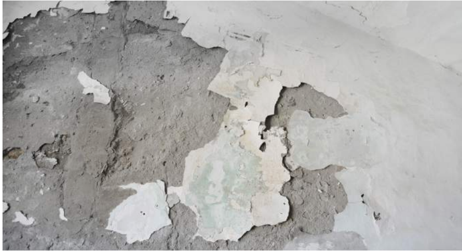
Fig.142 Interior wall decaying
