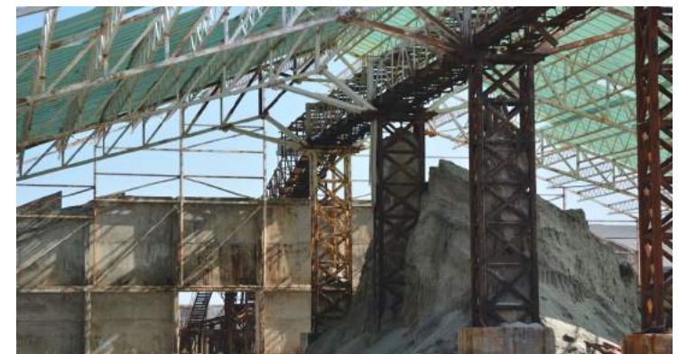
Fig.35 Decaying sat warehouse
