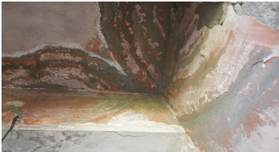
Fig.138 Mould and moisture damage on interior walls and ceiling
