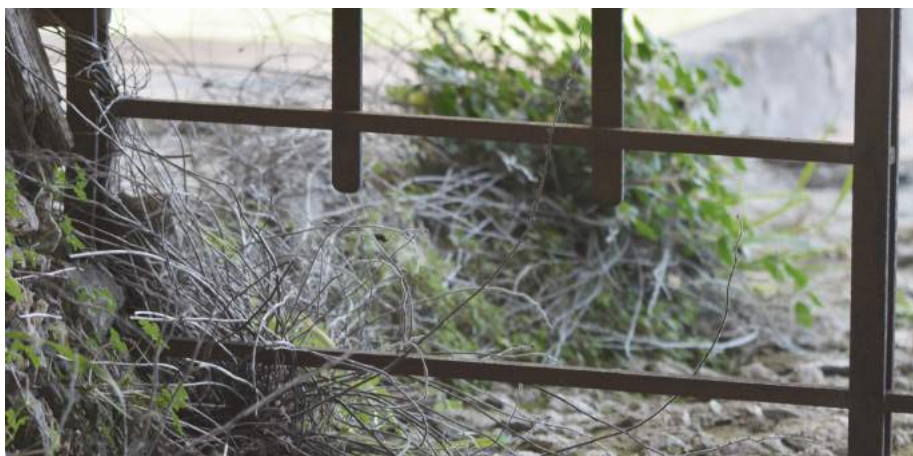
Fig.140 Vegetation overtaking the construction
