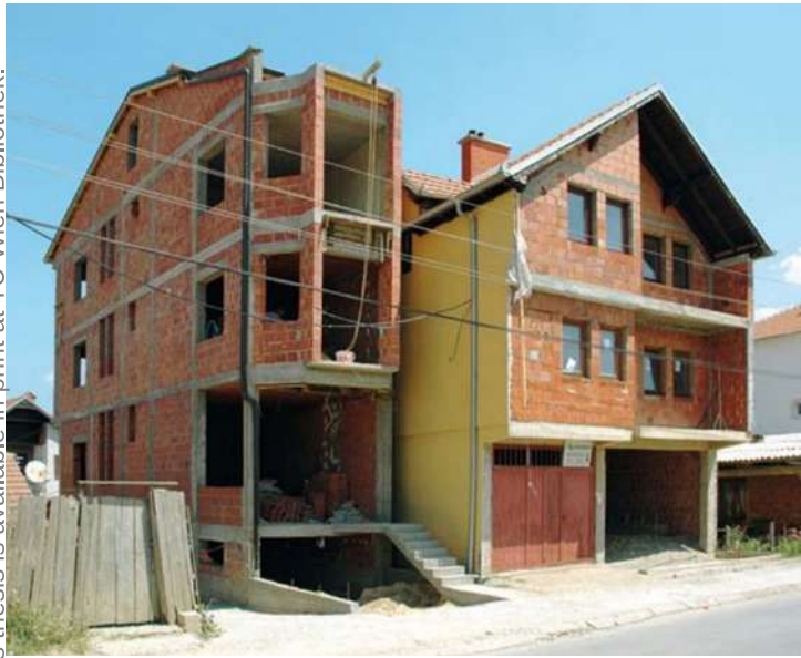
Figure 24: Houses facade appear not proper with each other.
