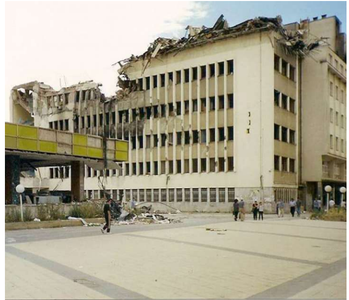
Figure 22: Old post office with demolished roof.
