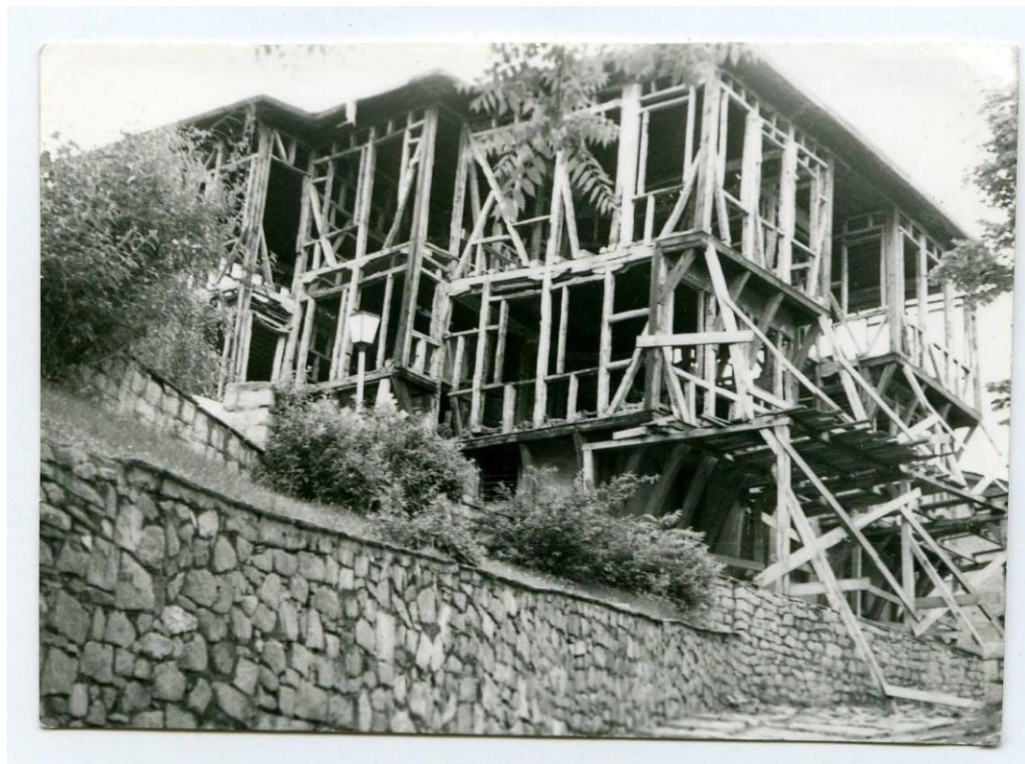
Figure 17 House of Georgi Mavridi - construction (Scanned photo from Bulgarian national institute of cultural heritage)
