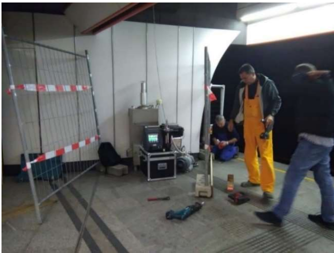
Figure 2.1 Employees of the Wiener Linien setting up the grid wall around the measurement setup at station Stubentor U3
