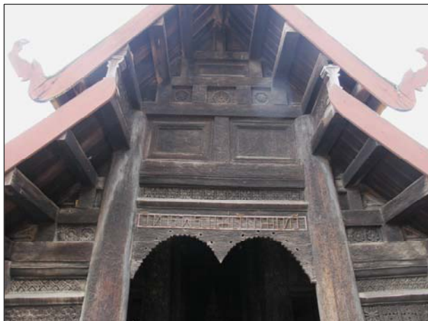
Fig. 3.45 First transverse frame at the frontal facade; we can observe that the second and third aisle beams mortised directly to the nave pillars
