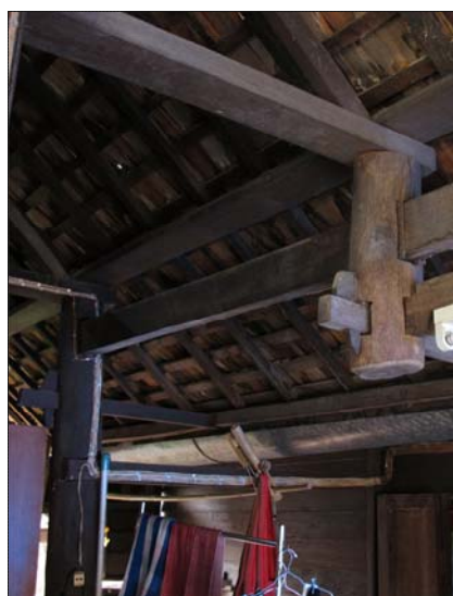
Fig. 4.14 Carpenter assembled crosswise beam and purlin face upside; they are carried by a hanging post
