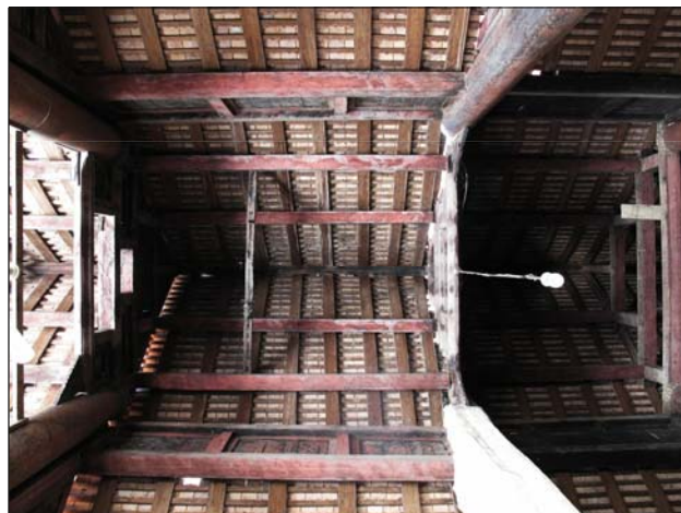
Fig. 3.30 Purlins from the second bay meeting the third transverse frame in nave roof
