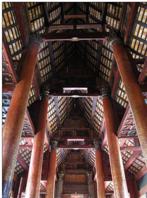
Fig. 3.54 A view from principal hall towards the first transverse frame presenting the roof structure
