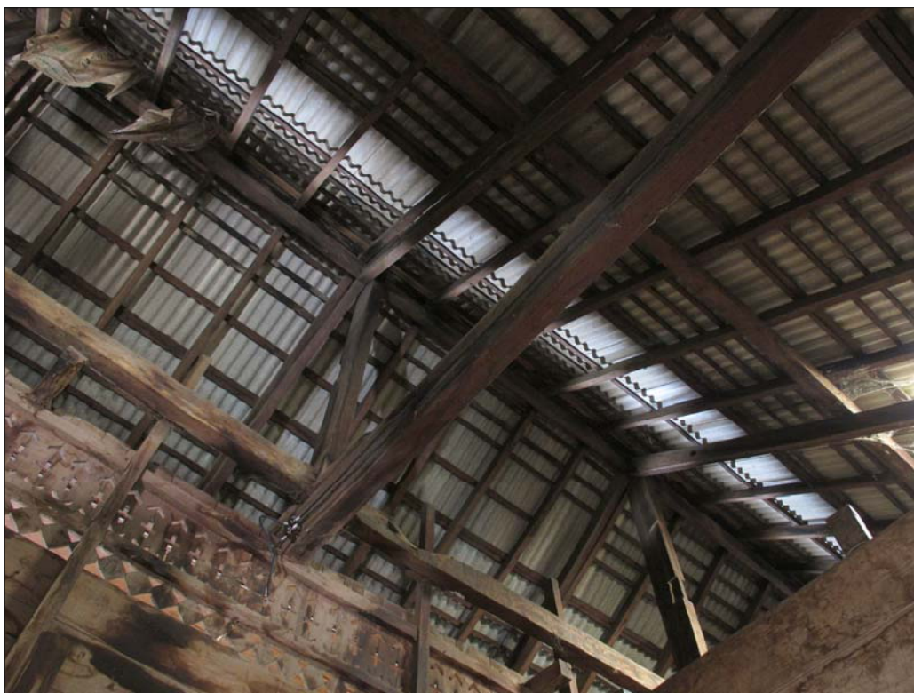
Fig. 4.46 combination of tang yo and rafter in the roof structure of the monk residence at Baan Luk monastery
