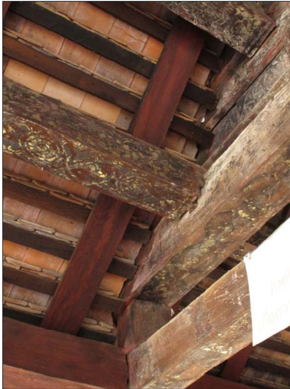
Fig. 5.38 The fastening of purlin using recessed dovetailed shape also found in Lan Na region, a sample from the viharn of Lai Hin Luang, Lampang province
