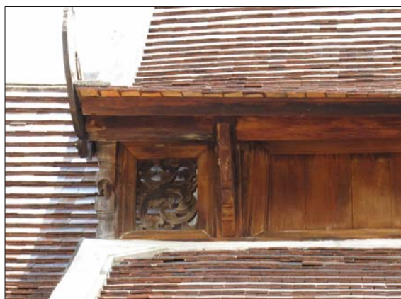
Fig. 2.17 The cantilevering purlin's edge or " hua pae " as mentioned in building treatise Nr.6; a sample from the viharn of Ton Kwen monastery, Hang Dong district, Chiang Mai province
