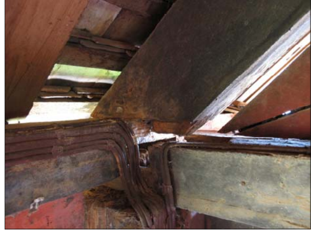
Fig. 4.37 curved tang yo at aisle roof rests partly on beam and partly on main purlin; the photograph shows deterioration of the joinery
