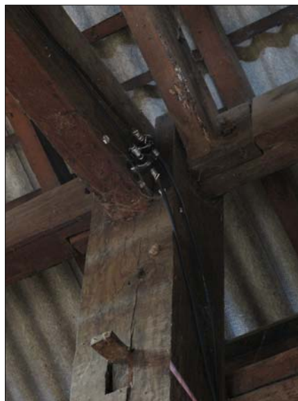
Fig. 4.48 Carpenter detached tang yo from the tie beam and placed it on lengthwise beam
