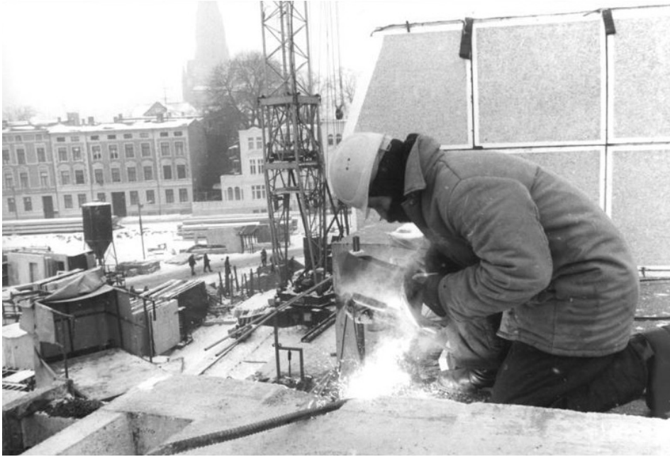
Figure 10. Plan welder at work in Schwerin's inner-city new construction and reconstruction area "Großer Moor." Pre-heated concrete elements and steel wires for welding, made it possible to rapidly assemble at temperatures below minus 15 degrees. Sand, water and cement were also kept above freezing in special containers.
