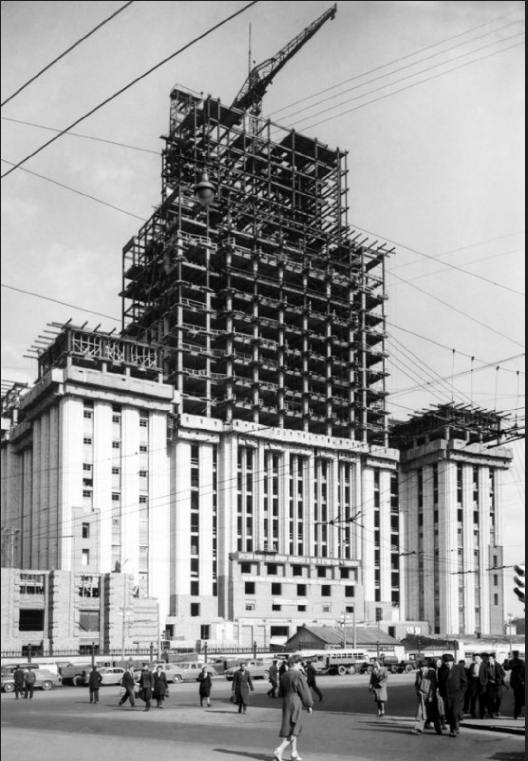
Figure 31. (this page) Construction of the Ministry of Foreign Affairs in Moscow Figure 32. (page right) Contrasts of 1950s: A courtyard near the Kiev Train Station
