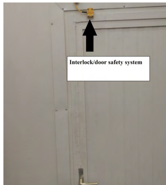
Figure 3.15: Interlock on the doors to avoid the Level 4 class laser's direct meeting with human skin or eyes. Source [5]
