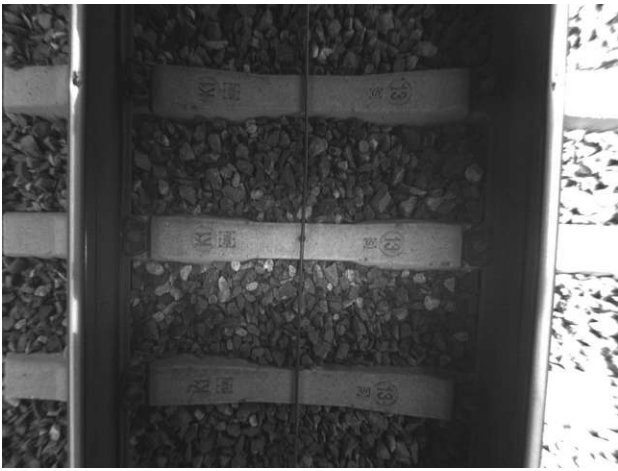
(a) Rail damages are of particular interest for maintenance.
