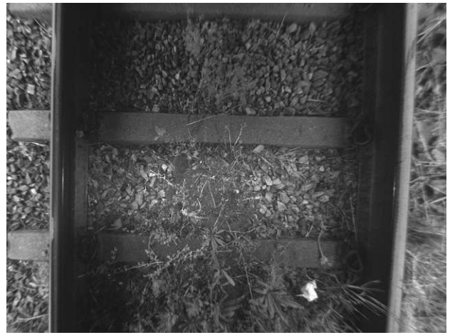
(b) Heavy vegetation on the trackbed and next to the rails.
