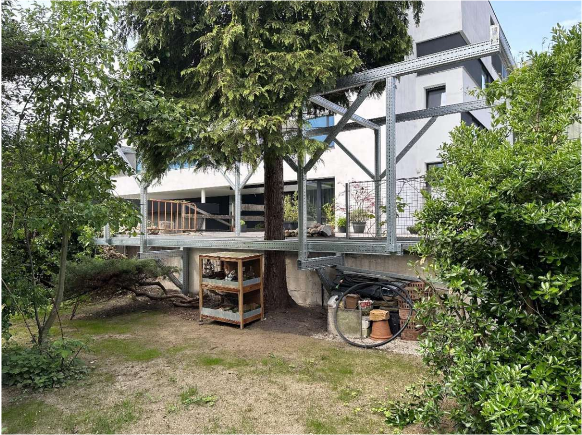
Figure 90: P4 - Change in level of the terrain – two cantilevers support the structure.
