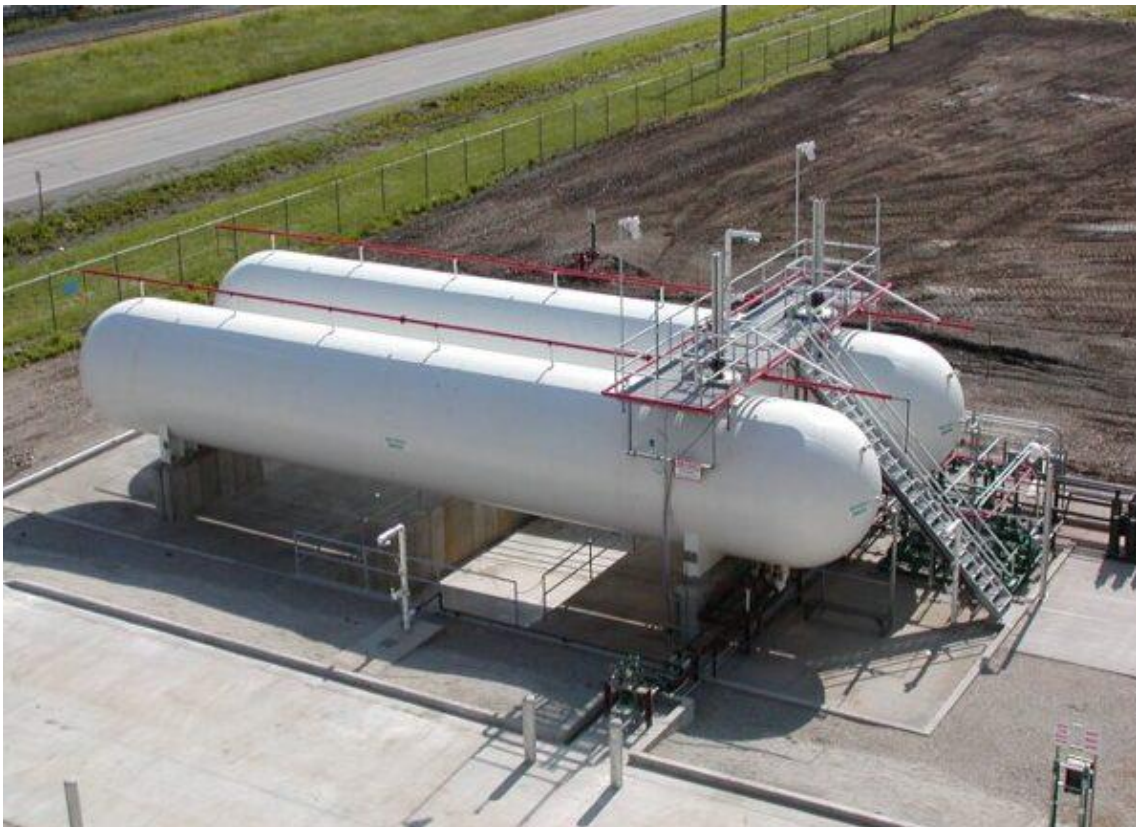
Figure 20 Ammonia storage tank. Retrieved from (“Ammonia Storage Tanks - Sagebrush” 2020)
