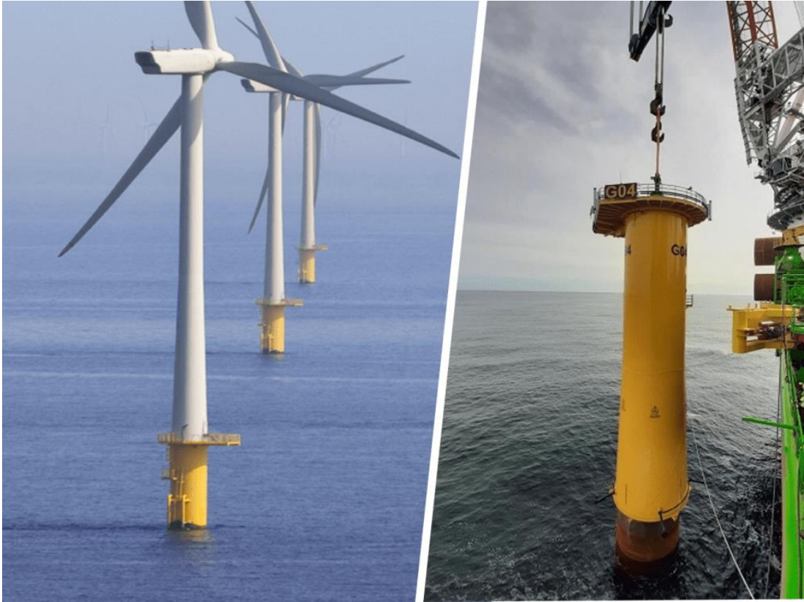
Figure 9 Monopile foundation for offshore wind turbine. Retrieved from (“Offshore Wind Turbine Foundations: Leveling and Fixation with Hydraulic Cylinders” 2022)
